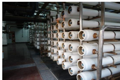
Reverse Osmosis Plant
