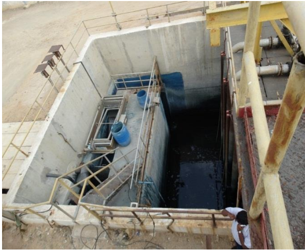
Lifting Pump station
