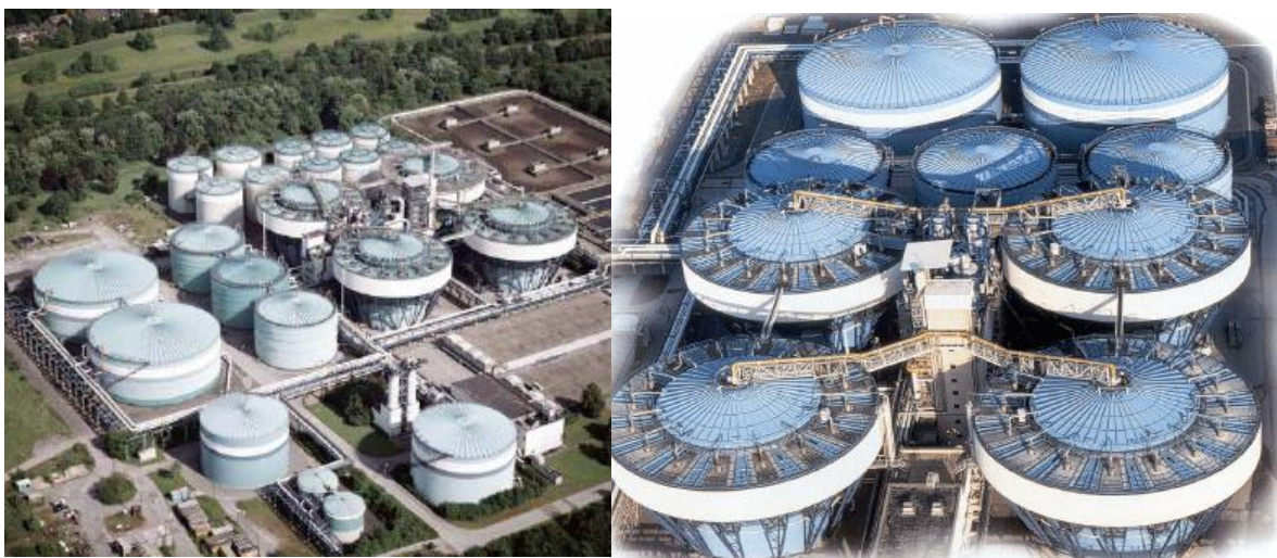
Fig. no. 6.17- View of tower biology system at Chempark Leverkusen
